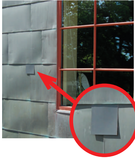
ContinentalBronze shown in contrast to a naturally aged copper wall with 4+ years of exposure.
